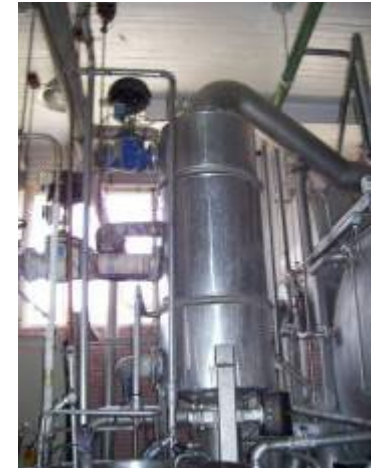
Hot water heater
