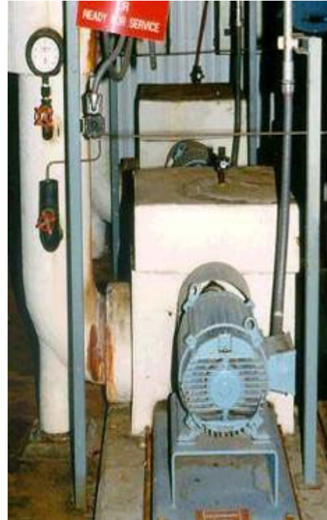
Combined motor & pump efficiency = 59%
