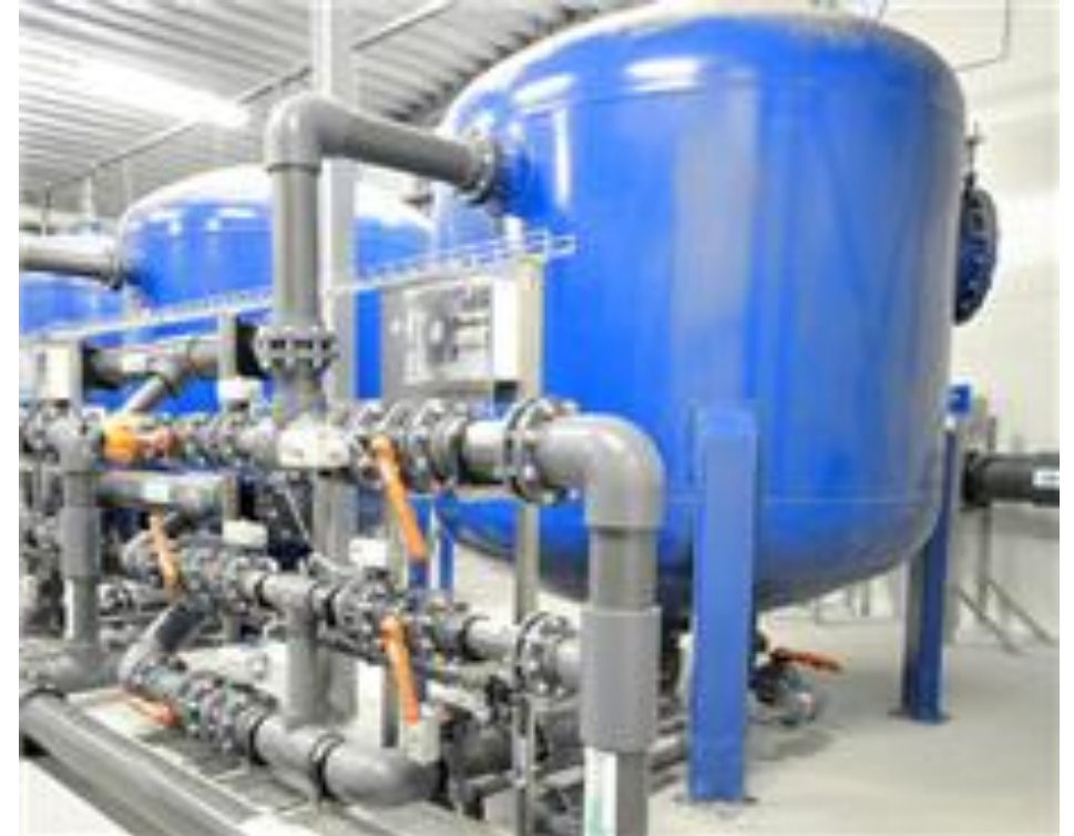
Chemical treatment with automated monitoring and control
