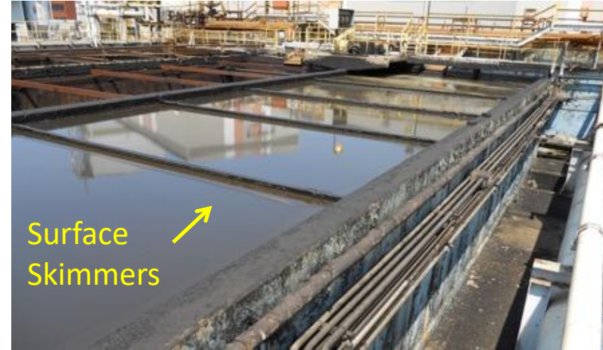
Settling/Separation tanks (chemical treatment)
