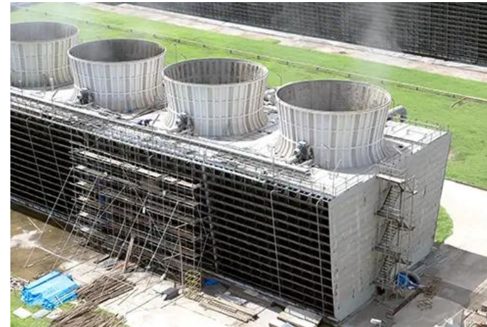
Cooling tower showing water loss through evaporation
