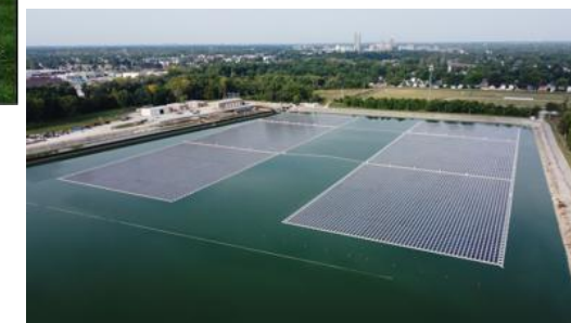
Floating Solar Array (Photo Courtesy of WPCP)
