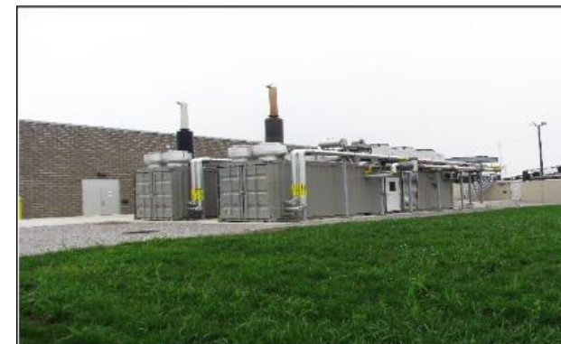
Two 400kW Engine Driven CHP Systems w/ Heat Recovery (Photo Courtesy of WPCP)
