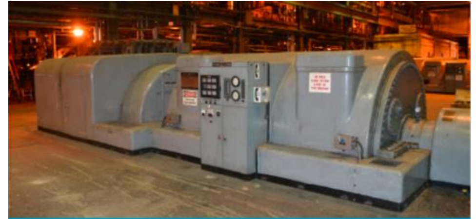
Steam turbine CHP installation at an industrial facility in New York. Photo courtesy of Recycled Energy Development
