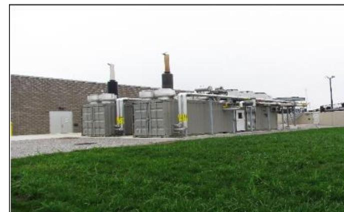
Two 400kW Engine Driven CHP Systems w/ Heat Recovery (Photo Courtesy of WPCP)
