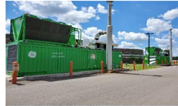
CHP Units 1 and 2 – Total 1.26 MW Biogas Fueled Source: St. Cloud NEW Recovery Facility
