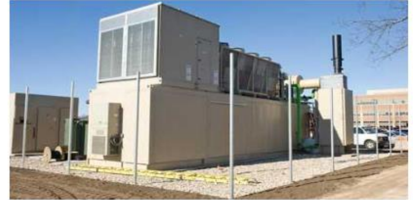
CHP Engine Generator Set with Heat Recovery and Gas Clean Up Source: DOE CHP TAP
