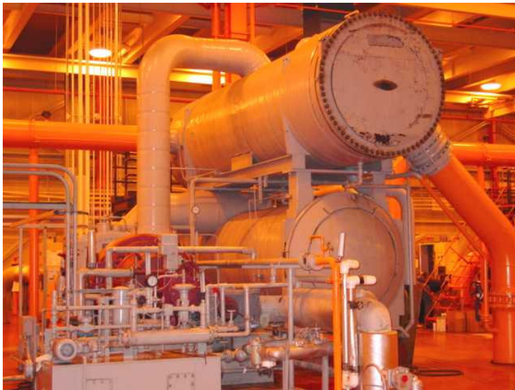
4,000 RT Steam Turbine Driven Chiller
