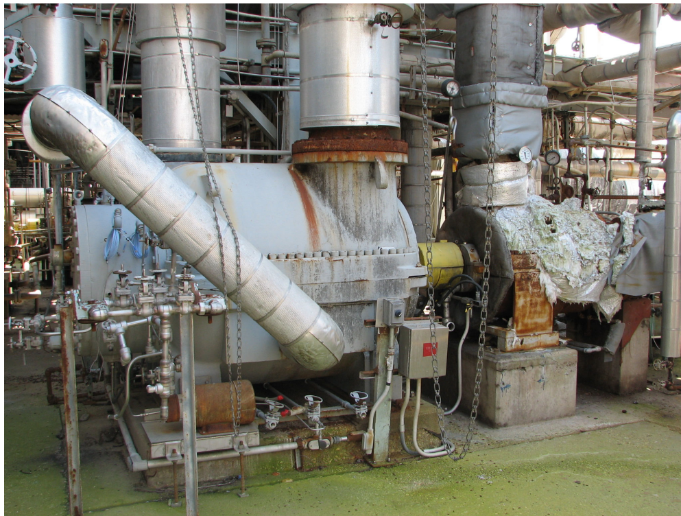
2-stage refrigeration (R134a) compressor
