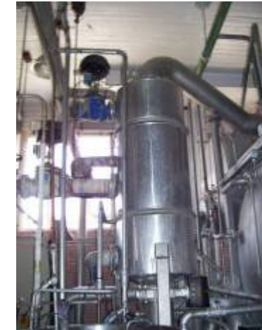
Hot water heater
