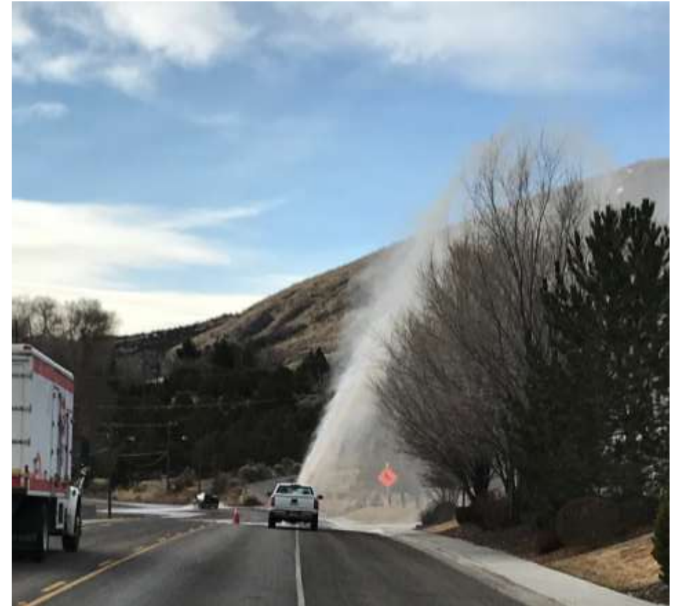
Leak on 12" main. Photo courtesy of Harold Hargaves, City of Pocatello, ID.
