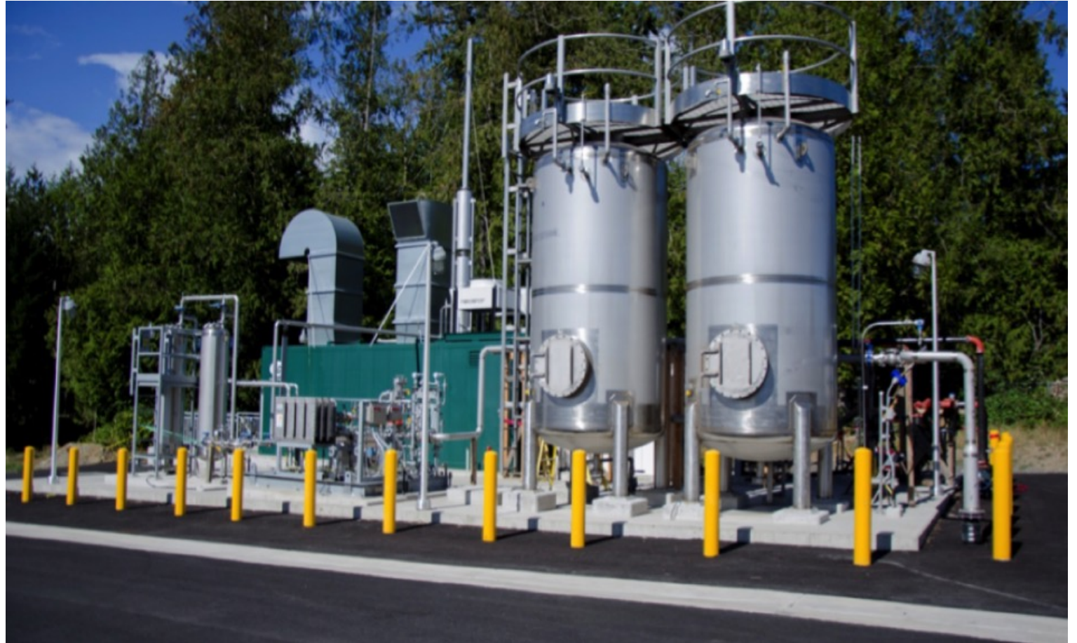
Biogas conditioning equipment for 250 kW CHP project at Central Kitsap WWTP, WA
