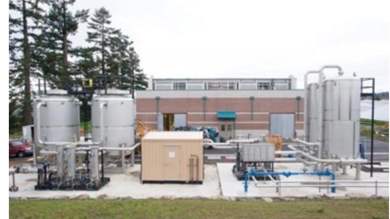
A Unison gas conditioning system is located outside of the CHP building
