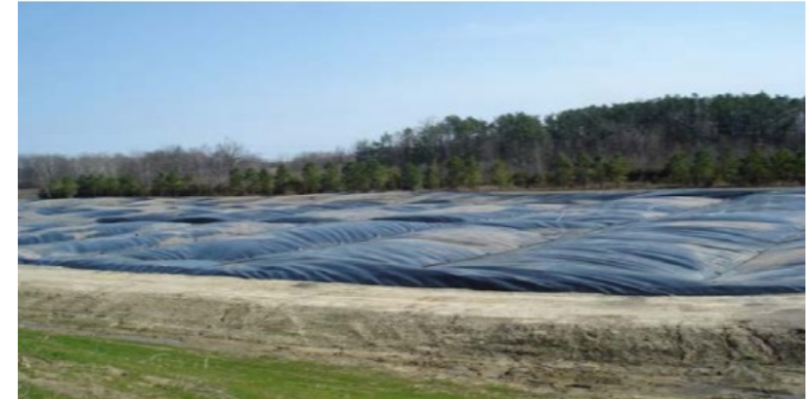
Covered lagoon anaerobic digester. The digester uses the waste Purdue produces by processing 1.2 million chickens weekly
