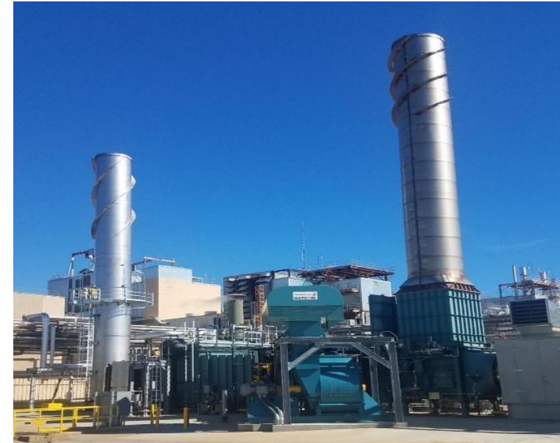
CHP System at Shaw Industries
