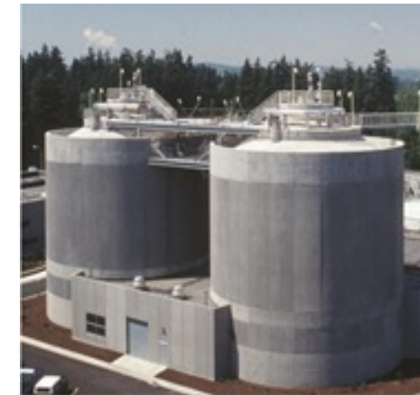
Two 70,000 gallon FOG storage tanks accept 100,000 gallons weekly of FOG
