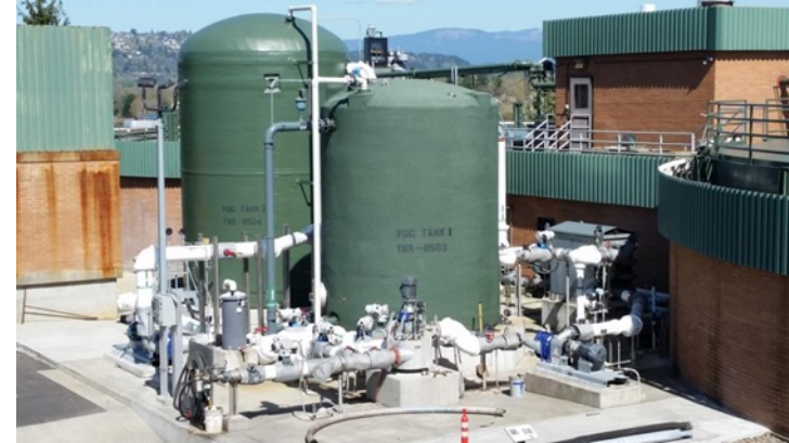
Delivered FOG is stored and blended in tanks, then metered into the digesters for co-digestion with sewage sludge
