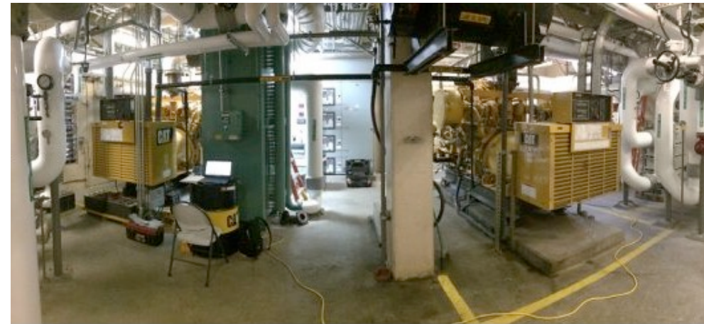
The Gresham WWTP produces 5.8 million kWh/year with its two 395 kW Caterpillar engines
