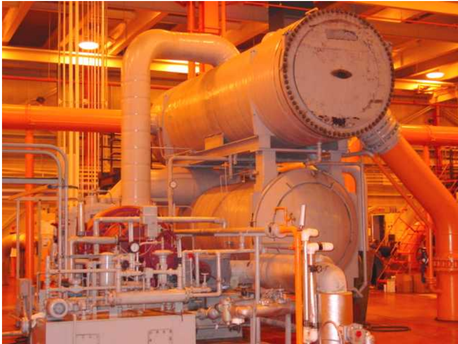
4,000 RT Steam Turbine Driven Chiller
